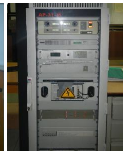
Figure 3: View of the control stand
